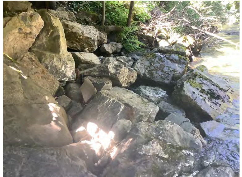
Mobilized riprap downstream left bank
