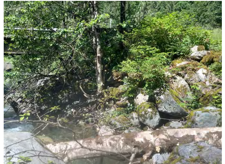
Scour right bank upstream
